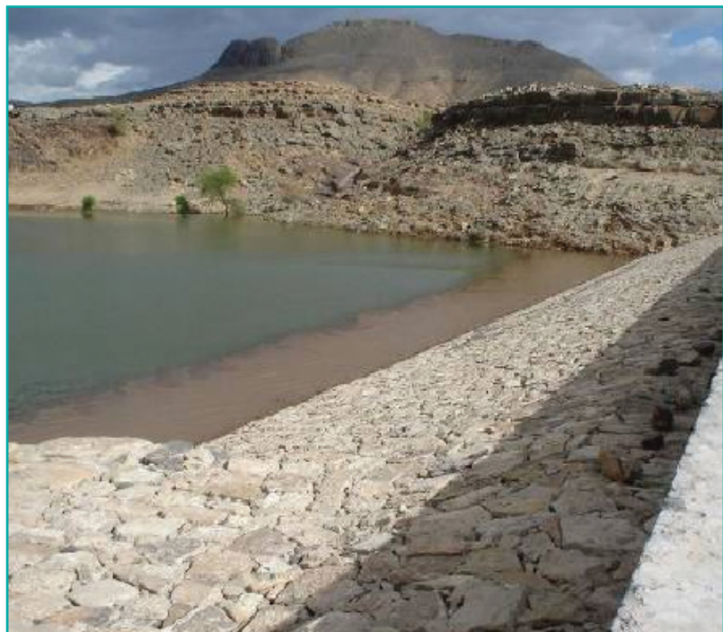
Figure 1. The Bani Naji Dam in Yemen was recently revitalised as part of a Halcrow contract to refurbish and design dams and improve water reliability where water supply depends greatly on groundwater sources.
