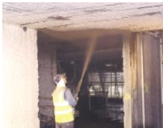
Figure 7: Application of sprayed concrete to repair a fire-damaged slab soffit following removal of fire-damaged concrete.
