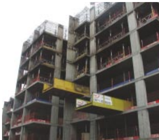
Figure 2: The concrete frame of a ten-storey building that was fire-damaged during construction.
